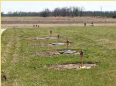
Runway 18-36 Threshold Lights and REILs
