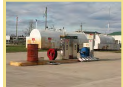
Fuel Farm, Card Reader and Pump Island
